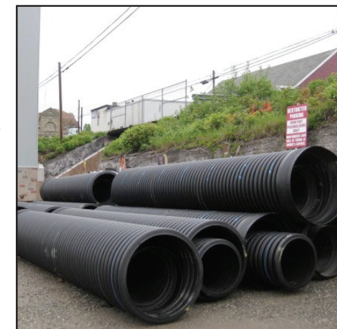
Large diameter corrugated HDPE pipe was easily maneuvered into place even in tight areas.
