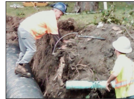
New Glasgow's combined sewer reduction project was on grade, on budget and on time.
