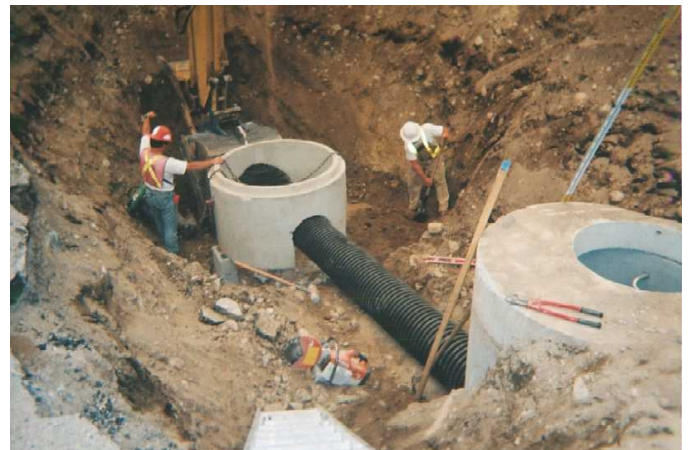
A two-man crew quickly positioned BOSS 2000 HDPE pipe for the ditch in-fill project.
