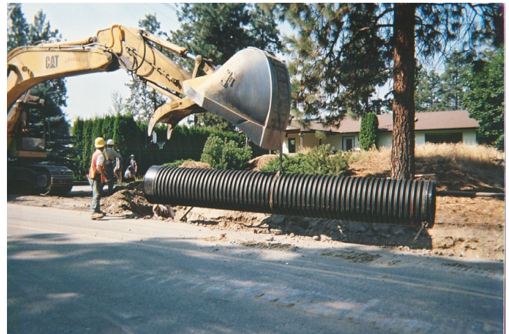
Easy to move, more than 400 meters of HDPE pipe was used for a water drainage upgrade project here.
