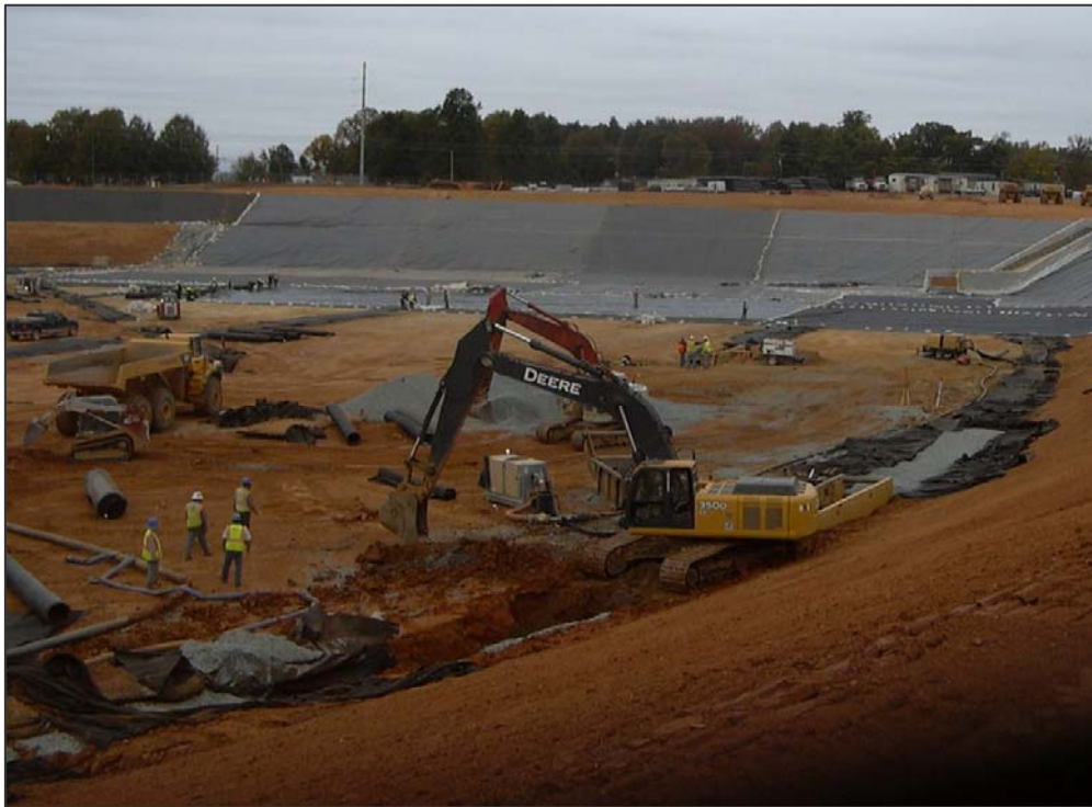
The Franklin Water Treatment Plant Reservoir Expansion project used corrugated HDPE pipe to create an underdrain system that will protect the geotextile liner. The 27-acre site was excavated to a depth of 30 feet. More than 14,600 feet of pipe was used for the project which was recently named Project of the Year by the Plastics Pipe Institute.
