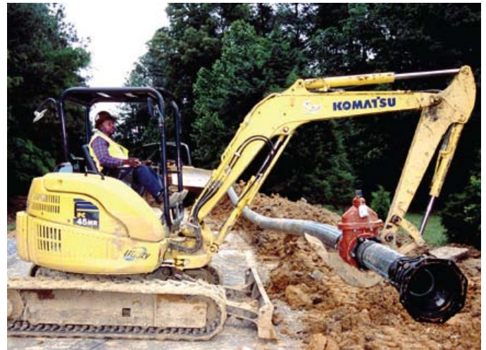
Fast and leak-free installation of HDPE pipe enabled Dalton to quickly add revenue from new services.
