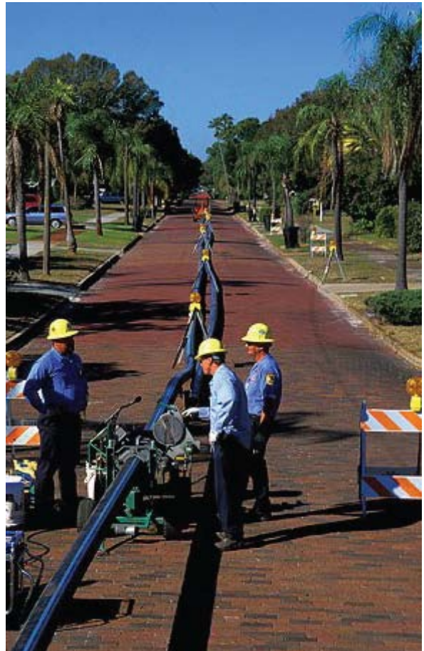
Leakless HDPE pipe being fused to form a jointless monolithic water main system in St. Petersburg.
