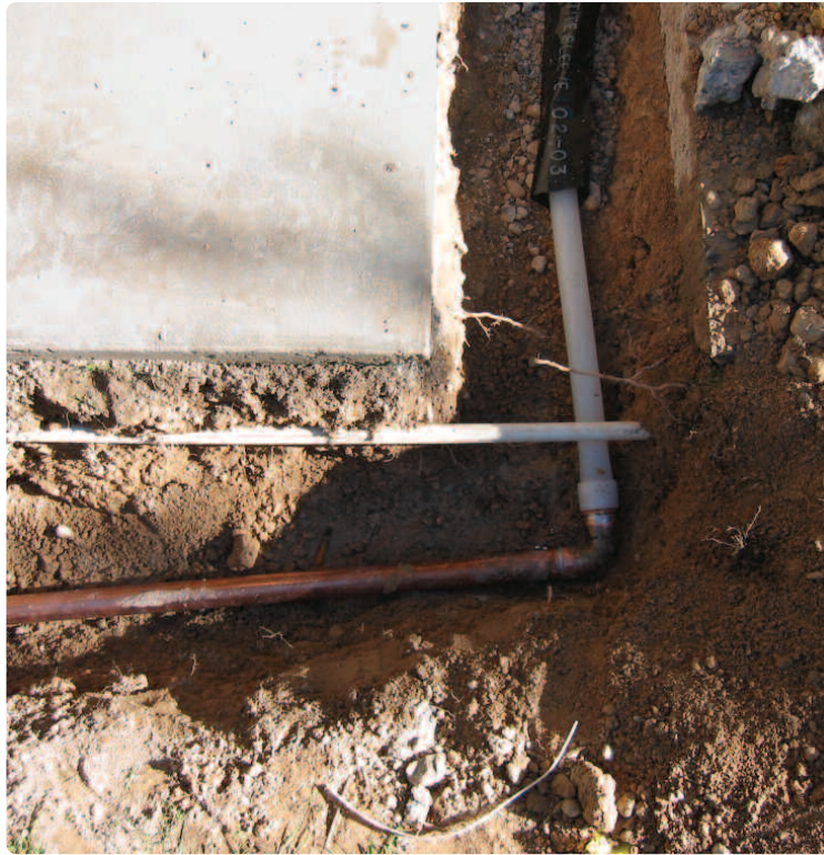
Uponor's Wirbo AQUAPEX tubing replaced copper pipe that was damaged in the acidic soil of Las Vegas.
