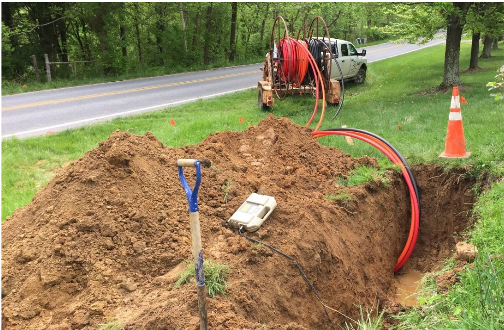
Figure 21 - PE conduit being dispensed from the top of a 3-way segmented reel to minimize the bend radius; conduit is installed using horizontal directional drilling (HDD).
