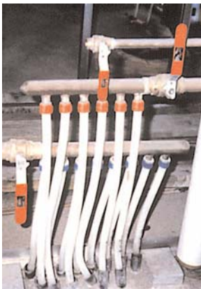
Manifolds supply hot and cold water to fixture in
