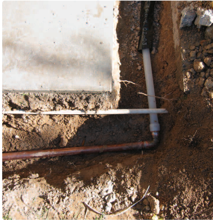
Uponor's Wirbo AQUAPEX tubing replaced copper pipe that was damaged in the acidic soil of Las Vegas.
