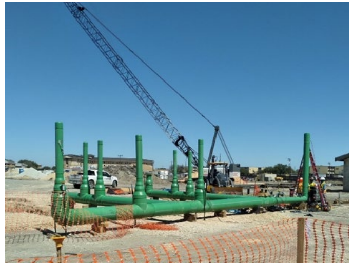
The Air Force's new basic training facility required large diameter pipe and fittings to move 155°F (68°C) water effectively throughout the campus at 90 psi. Using PP-RCT pipe also enabled sections of the system to be fabricated and lifted into the trench. Photo courtesy of Asahi/America
