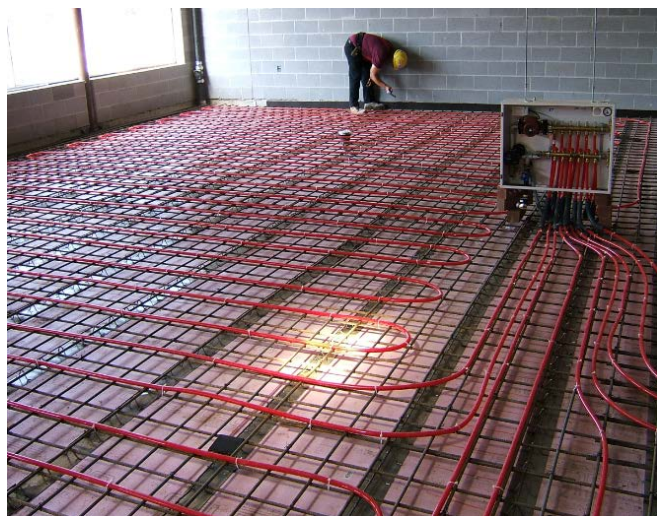
The system used nearly 20 miles of RAUPEX® 5/8-in. O 2 Barrier pipe and 42 PRO-BALANCE® manifolds. Photo courtesy Klimatrol
