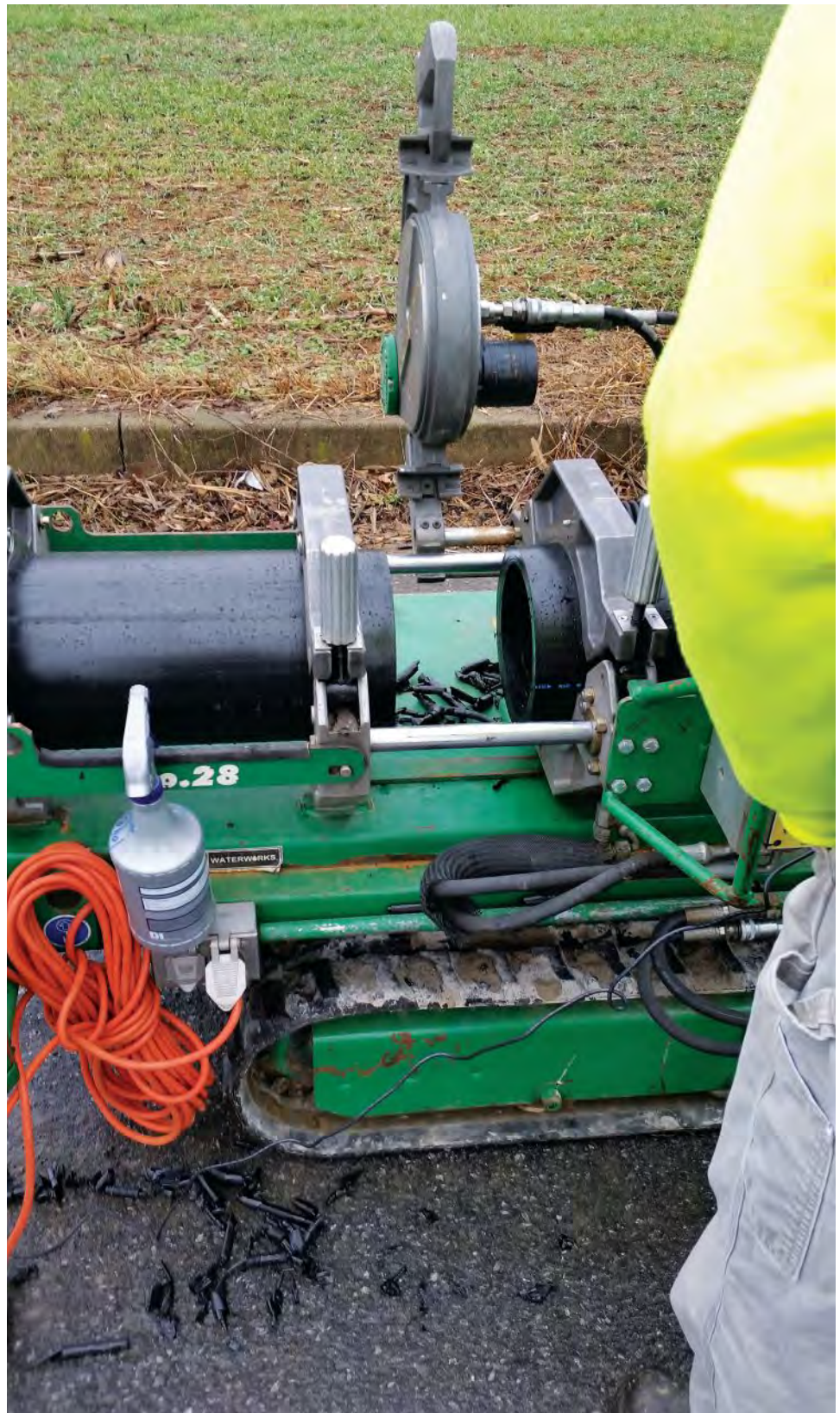
The HDPE pipe for the project was fused together in accordance with ASTM Standards F2620 and F3190 before it was installed with horizontal directional drilling.
