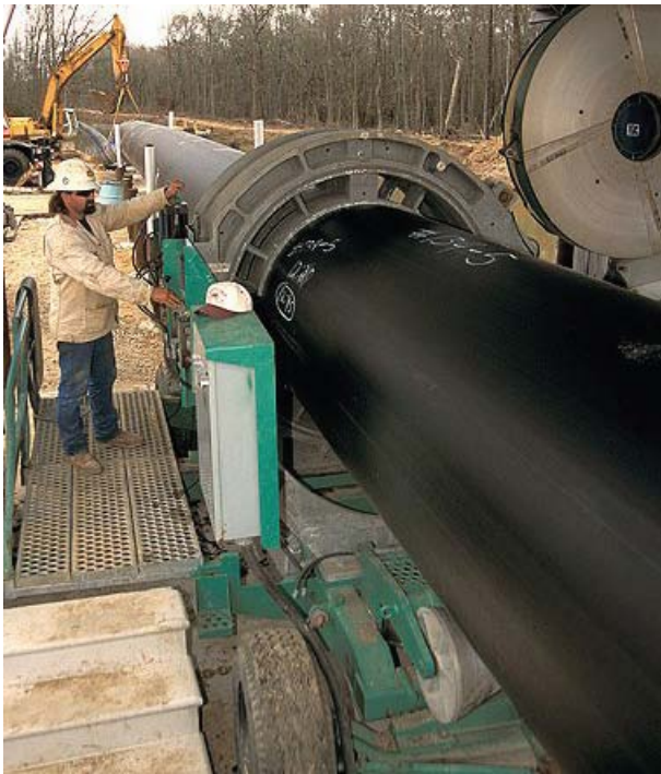
HDPE pipe being fused to join 48-inch diameter sections into a leak-free monolithic system.
