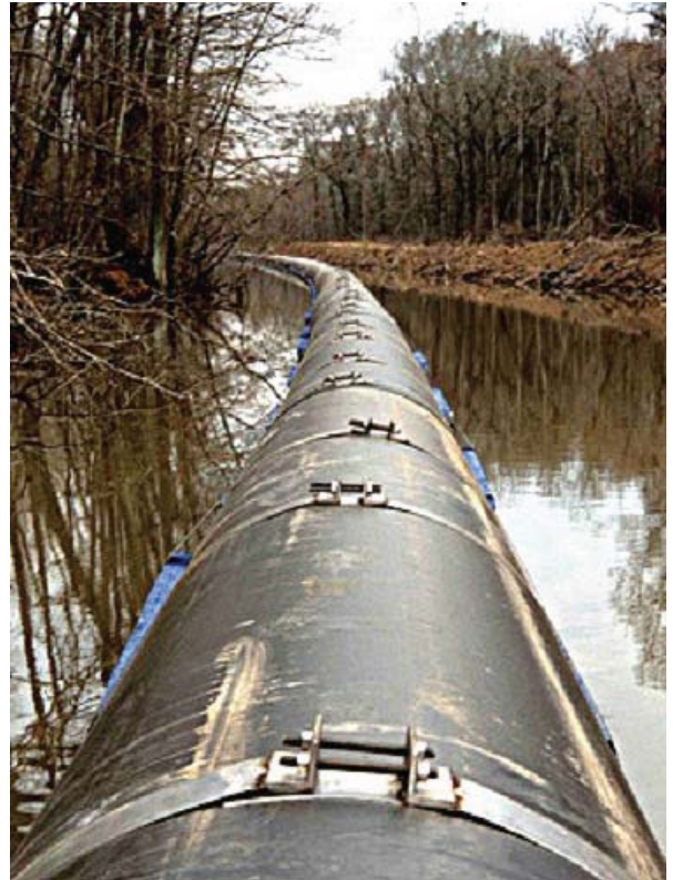
HDPE pipe with concrete ballasts attached to permit secure anchoring at bottom of Beaumont canal.
