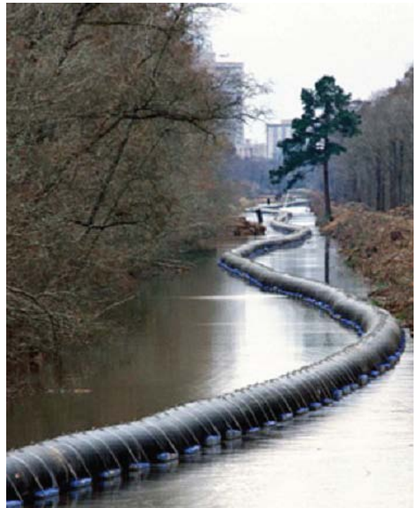
Flexible HDPE pipe is floated up a canal in Beaumont prior to submersion and installation with minimal impact.
