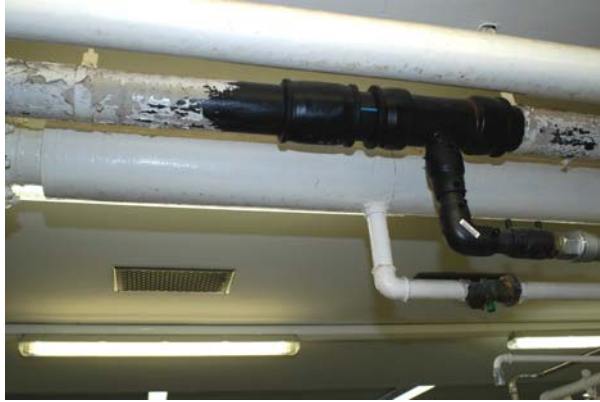
Fig. 6. Ceiling-mounted HDPE pipes in a changing and shower room built in 1961
