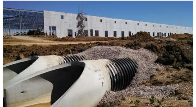
HDPE pipe connects to concrete aprons to provide an outlet for the system
