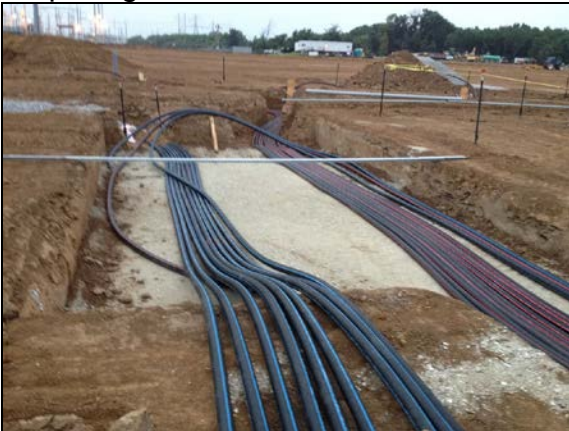
The O'Fallon solar farm used 19,000 feet of Cable in Conduit, which saved time and money.
