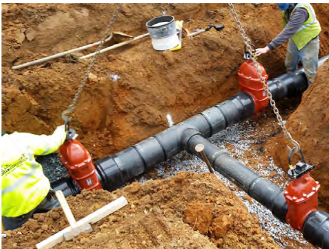
Shut off valves and fire hydrants were heat fused into the HDPE pipeline to further insure a leak-free, closed loop system.
