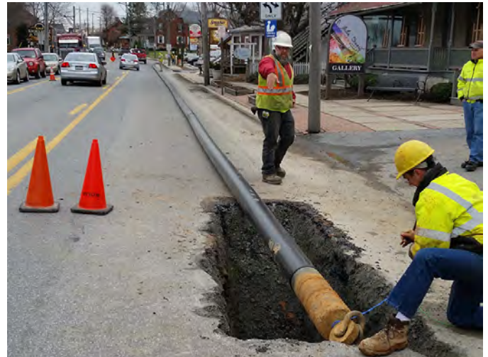
Horizontal directional drilling was used to install the new potable water pipeline for Intercourse, Pennsylvania. Nearly 10 miles of HDPE pipe was used.
