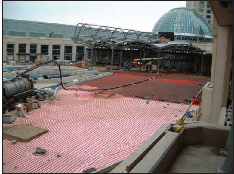
Figure 11.5 – Snow and Ice Melting in a Commercial Application
