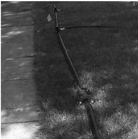
Figure 19 Example of Above Ground PE Bypass Pipe
