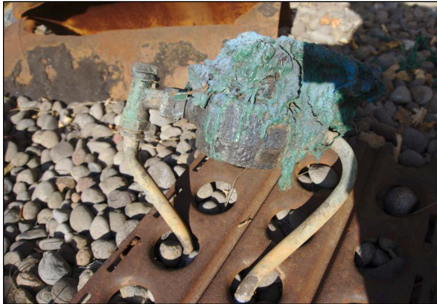
Figure 4: Damaged water meter
