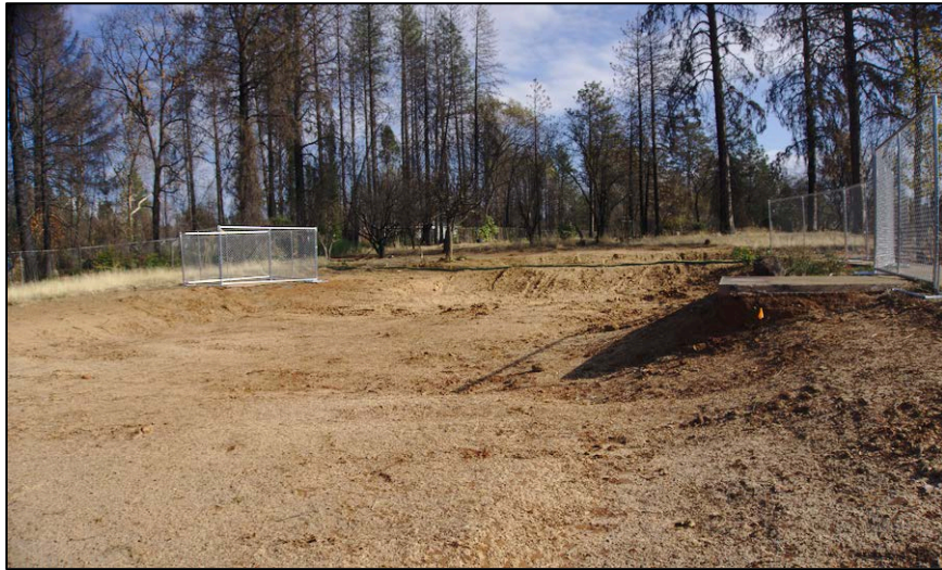
Figure 3: Site of a home after the fire; house debris and soil are removed
