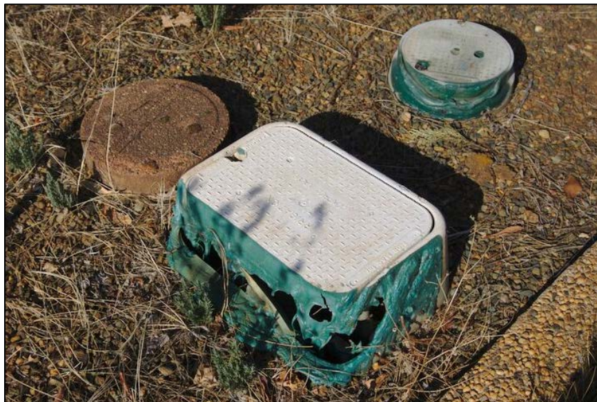
Figure 5: Partially melted meter box
